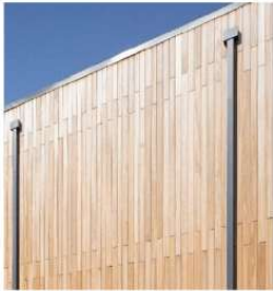
Example of: Timber Rainscreen Cladding (Photograph indicative) Treated Thermowood cladding to external walls. True type, size and layout to be developed
