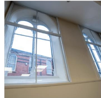
GRANADA SECONDARY GLAZING
